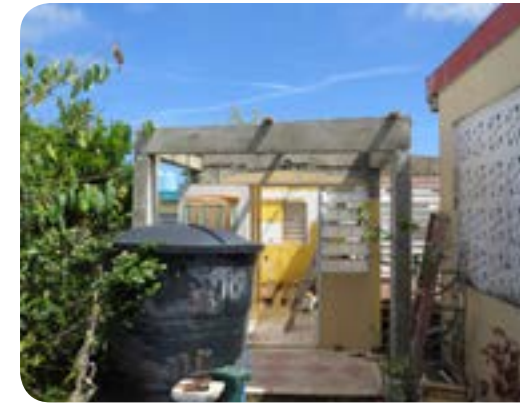
Ricky's home, before #ReconstruyeQ. Ricky is a hairdresser who supports his family and cares for his elderly parents. His apartment and the top level of his parents' home was destroyed in the storm.
